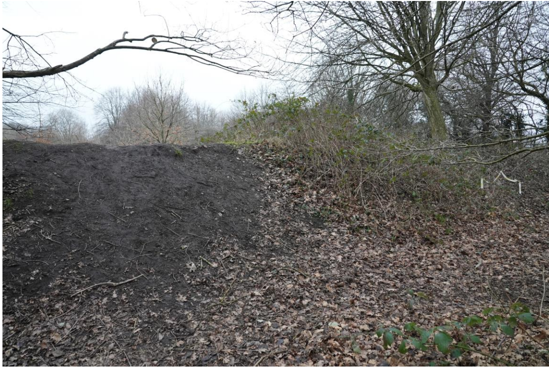
Photo 42: Image showing earth bank at TN10.
